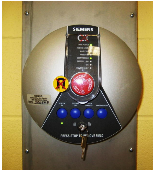
3T Control room Quench button
