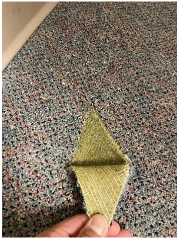
View of the carpet and mastic throughout several areas
